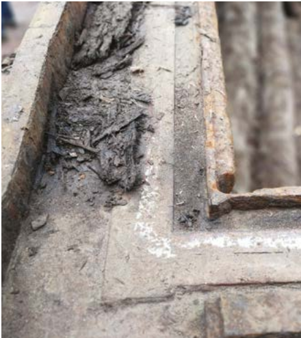
Drainage Opening Blocked
