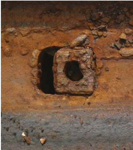
Cleat Badly Corroded
