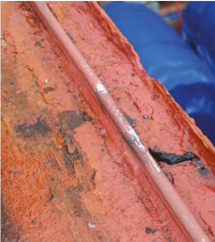
Drainage Channel Damaged
