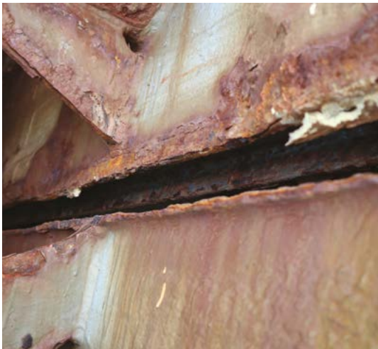
Gasket Partially Missing
