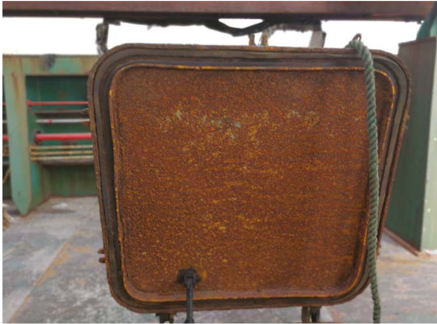
Rubber Seal on Hold Access Door in Poor Condition
