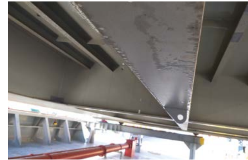
Single Skin Hatch Cover More Vulnerable to Sweat
