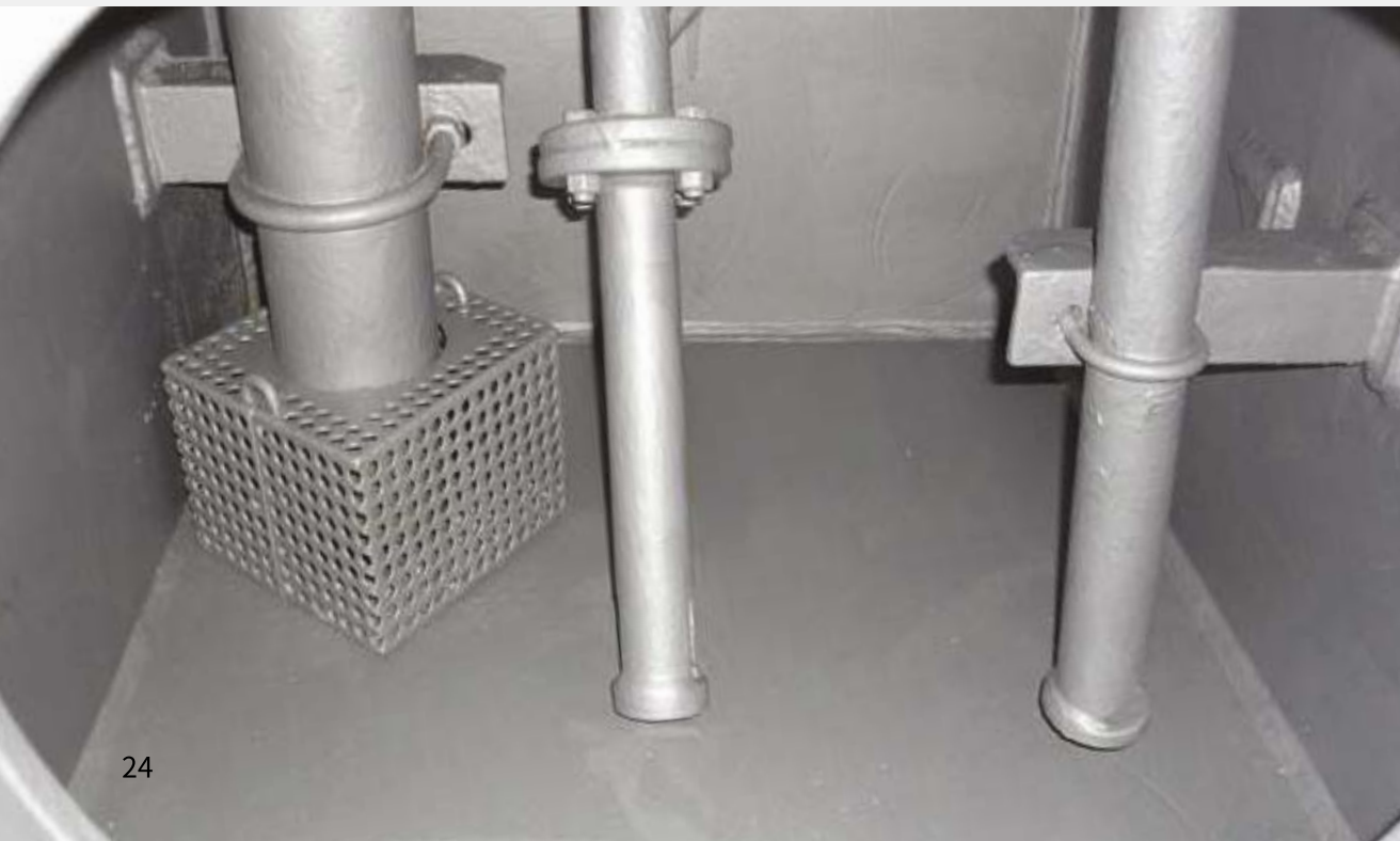
Inside a Bilge Well
