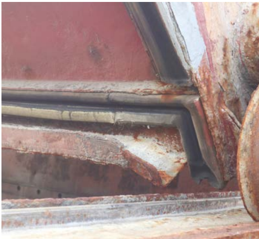
Gasket Permanently Distorted
