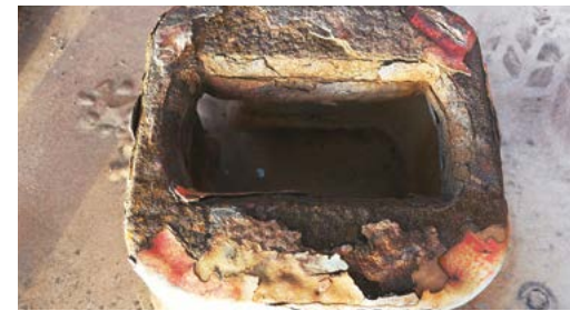
Seriously Corroded Socket
