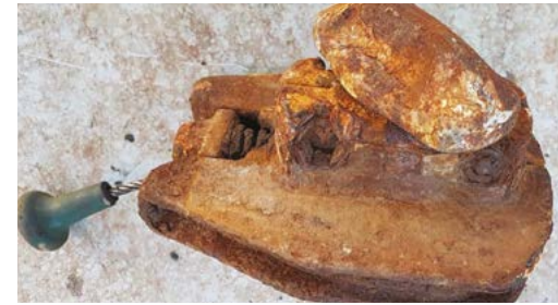
Seriously Corroded Twistlock
