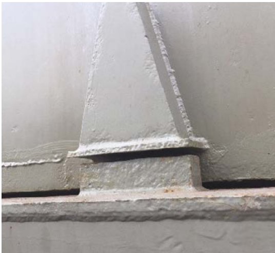
Weight of Hatch Covers All on the Gasket
