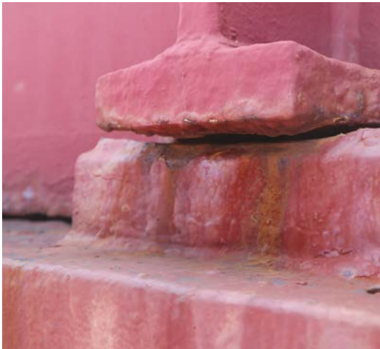
Worn Landing Pads
