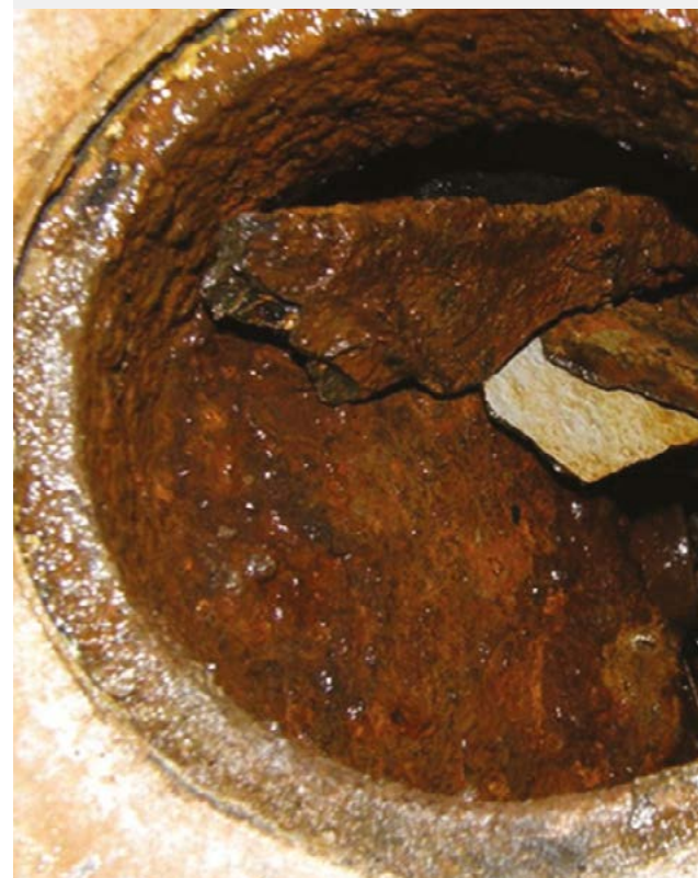
Non-Return Valve Clogged (Source: WOE)
